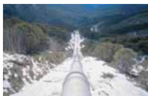
Southern Hydro's McKay Creek Power Station pipeline, in the Kiewa Scheme.
