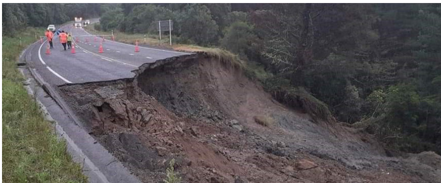
SH5 damaged by Cyclone Gabrielle.
