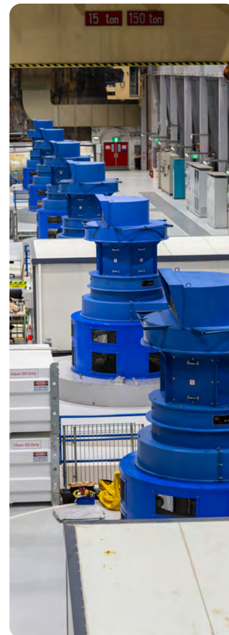
ABOVE: Manapōuri Power Station, Fiordland.
