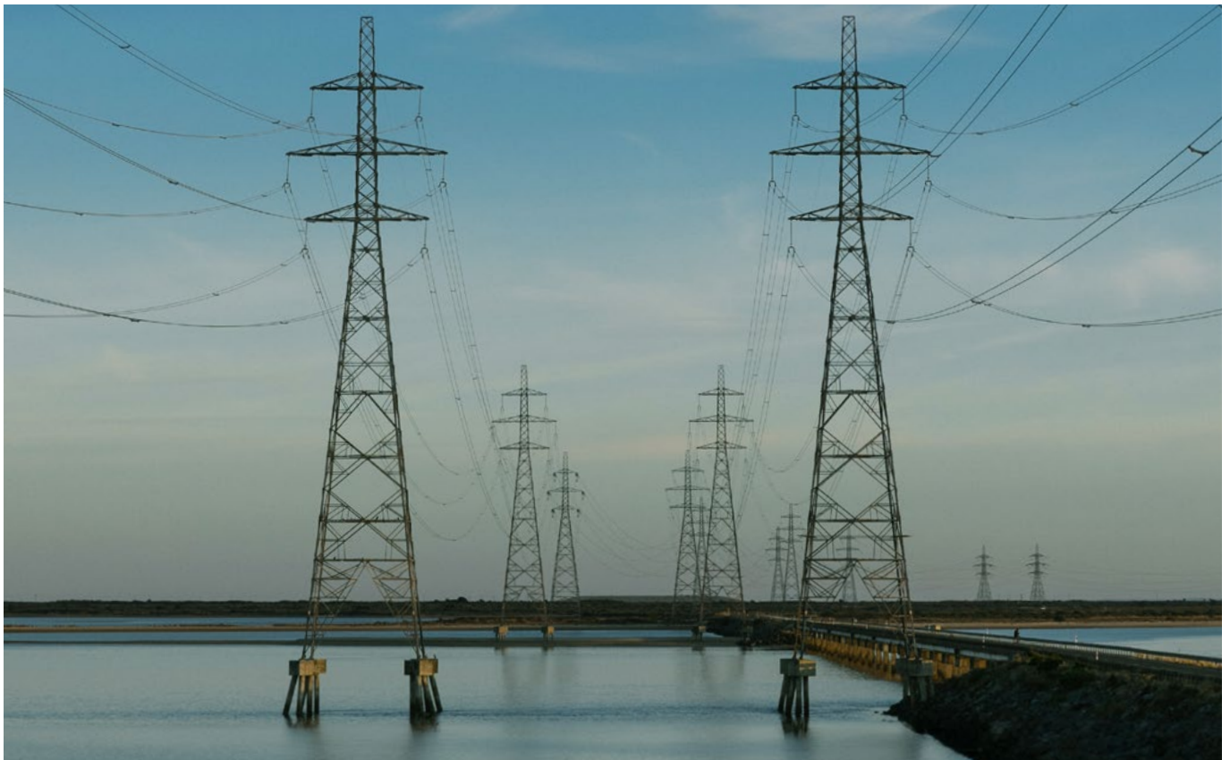
▼ Transmission lines in Southland.
