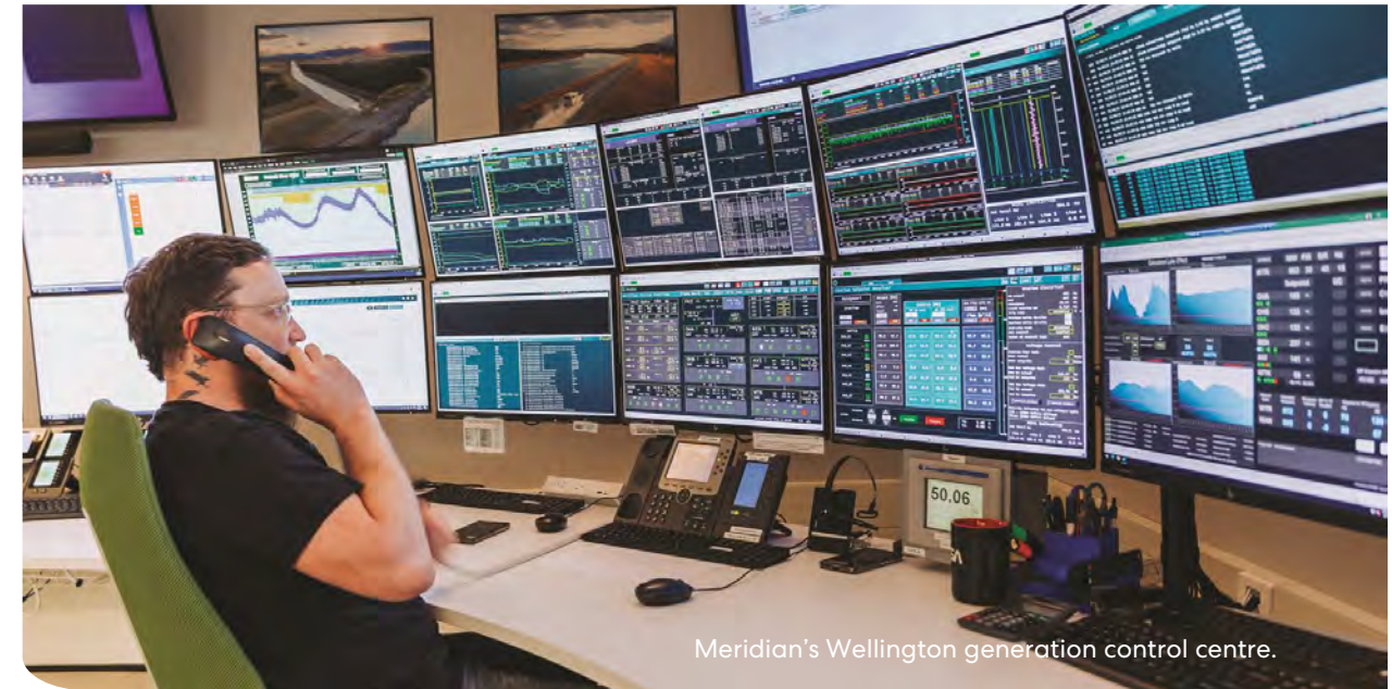
Waitaki Power Station control room.
