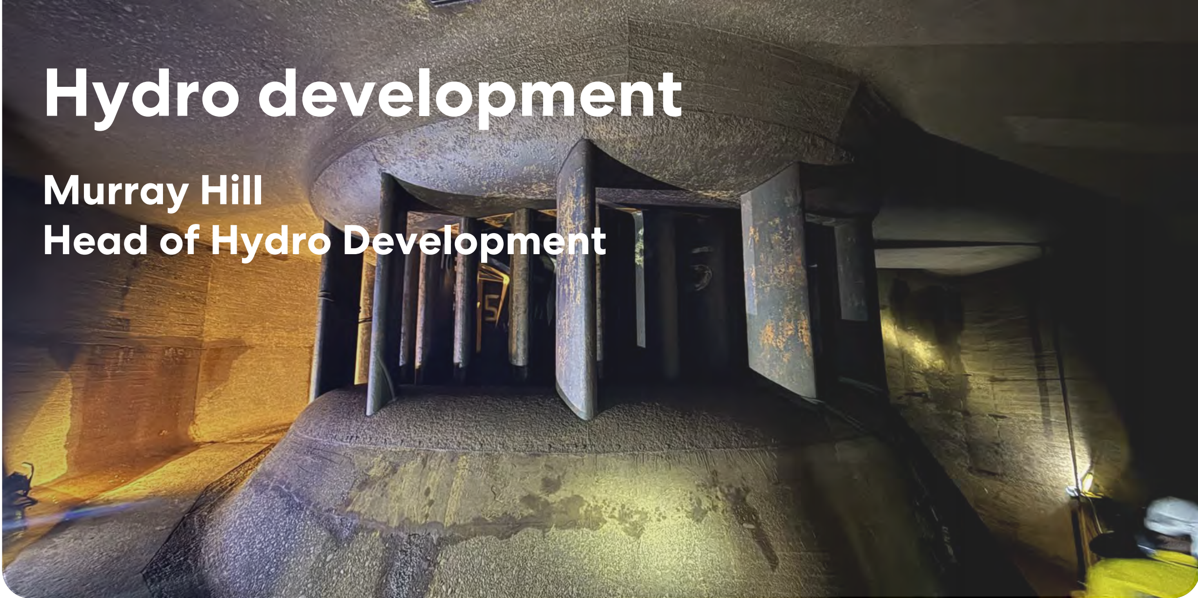
Waitaki Power Station – turbine inlet Unit 6.
