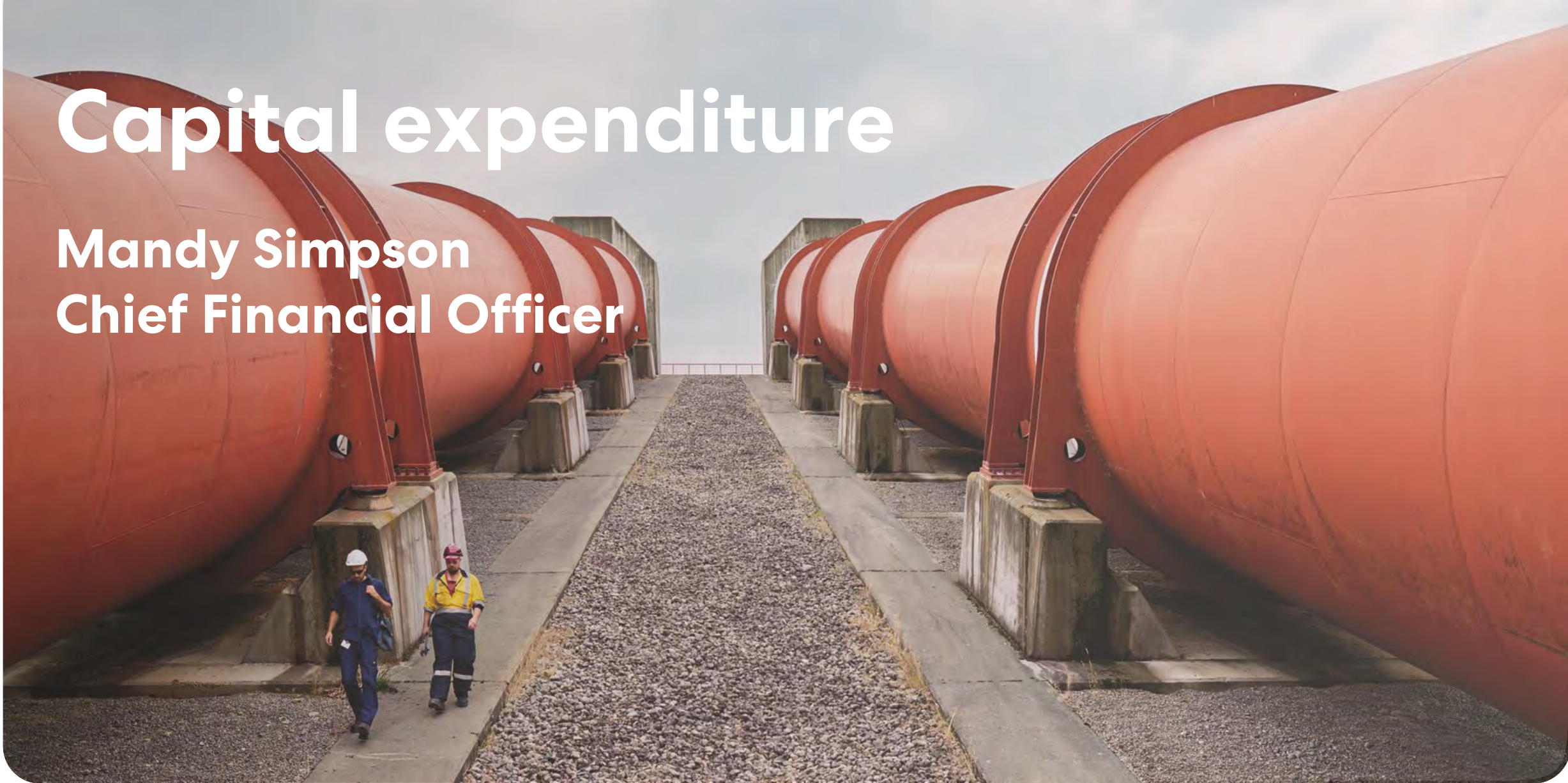
Penstocks at Ōhau A Power Station.
