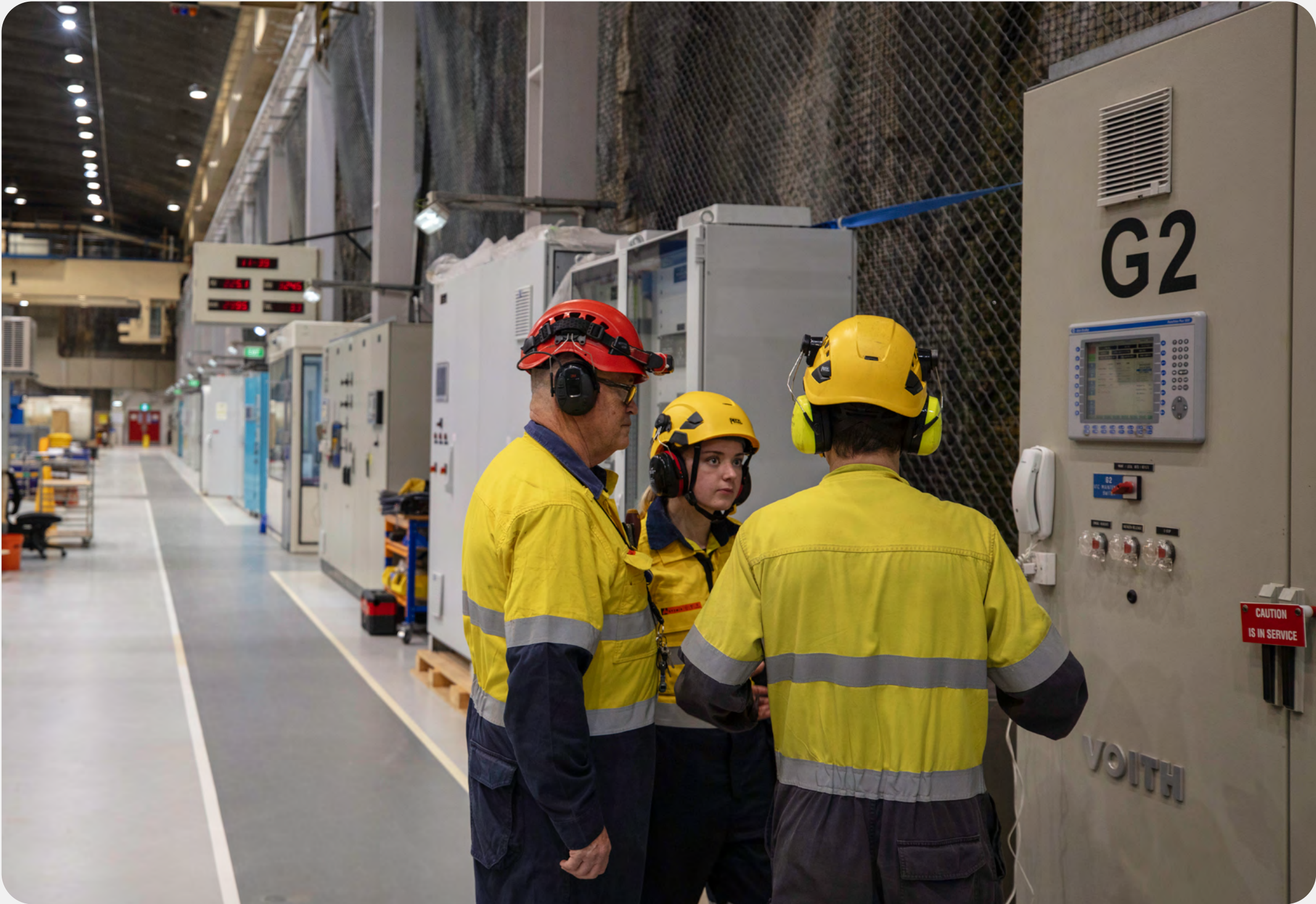
ABOVE: Manapouri Power Station, Fiordland.
